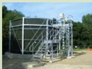
Typical HYRATE Polytower with Stairway and local control panel adjacent to doorway
