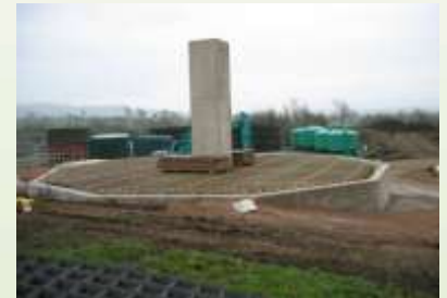
Timber matrix modules in place ready for construction of new HYRATE Polytower filter shell.
