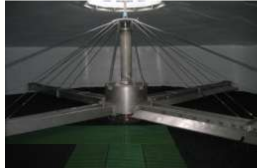
4 Arm all stainless HYCOVER trough type machine, to apply 55 lt/sec of primary sewage. Fitted with external over-mounted variable speed drive. Installed in an 11.75 mt HYRATE Polytower fitted with roof and low level odour extract system.
