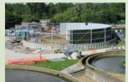
New 25 mt dia Polytower filter shell under construction using timber matrix as a working platform and for storage of materials.
