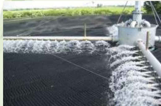
4 Arm motor driven HYCOVER tubular arm distributor applying some 170 lt/sec to 12.0 mt dia HYRATE nitrifying filter.
