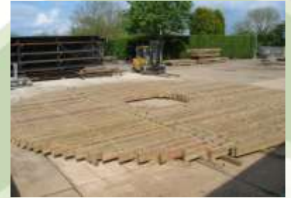
Factory check of pre-assembled timber matrix modules ready for loading onto delivery transport to site of new filter shell
