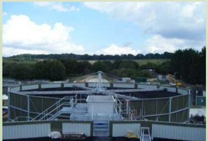
HYCOVER Distributors safely installed.
